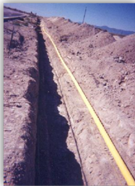
Natural gas is transported through underground pipelines throughout the U.S
